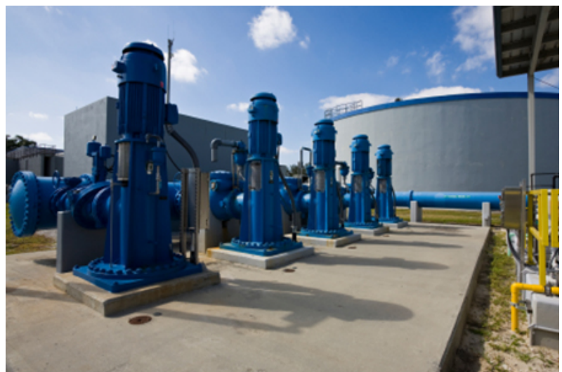
Fig. 2: At facilities such as water and wastewater pumping stations, there is a need for remote monitoring and robust diagnostic capabilities.
