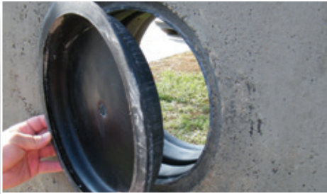
6. After concrete is cured, pry off the locator caps with a pry bar.
